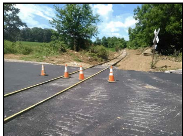
The almost completed Mt. Airy Road grade crossing in Shrewsbury, PA. Photo from Friends Facebook page.
