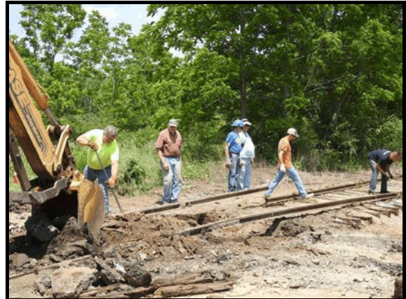
Our volunteers at work rebuilding the Mt. Airy Road grade crossing. Photo from Friends Facebook page.
